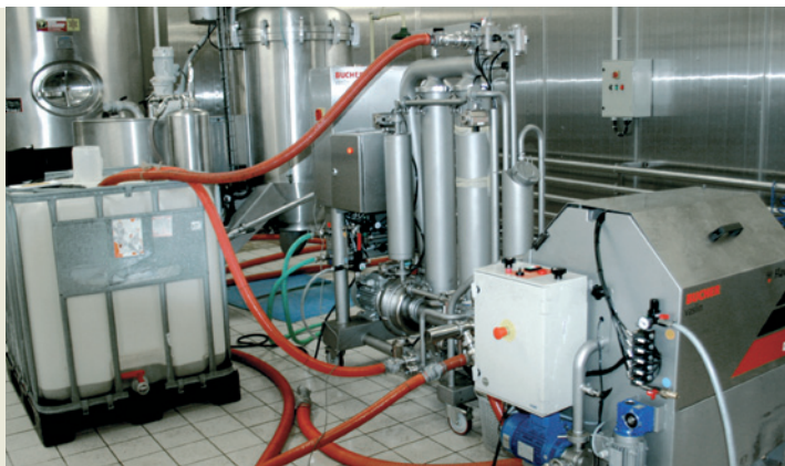
Juice lees filtration installation
