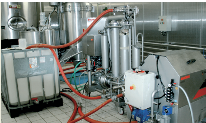
Juice lees filtration installation
