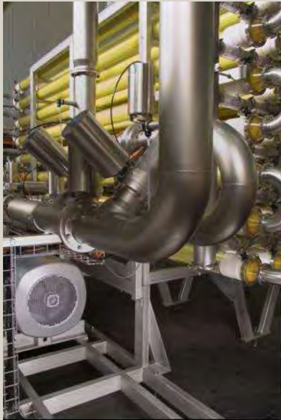
Pipes with valves
